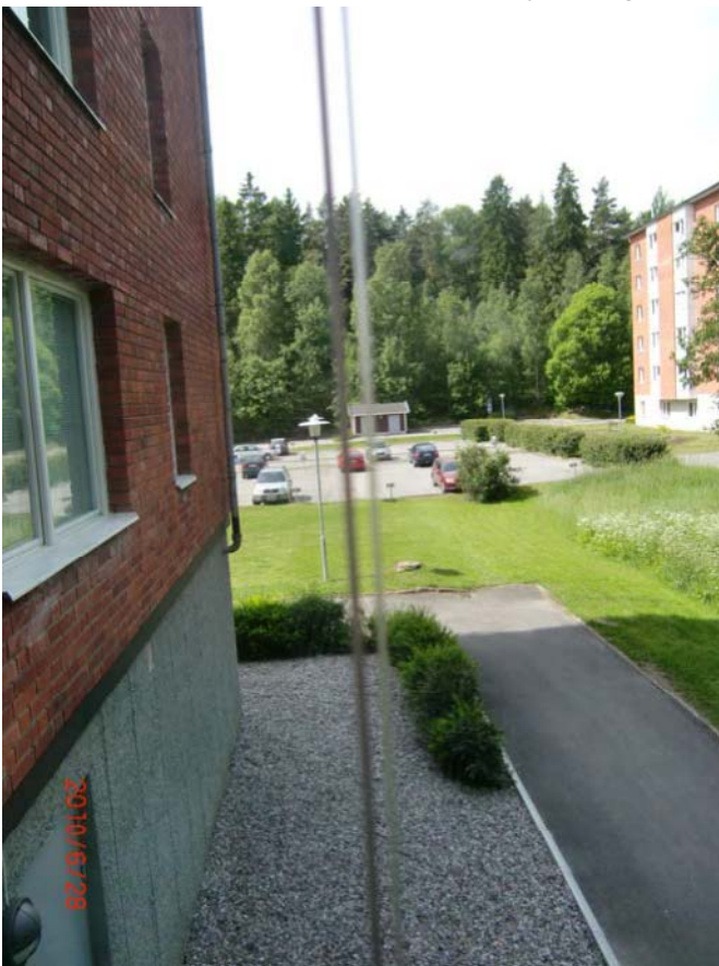
Picture 2. Gaps between panes of glass (Skogsviolen)
