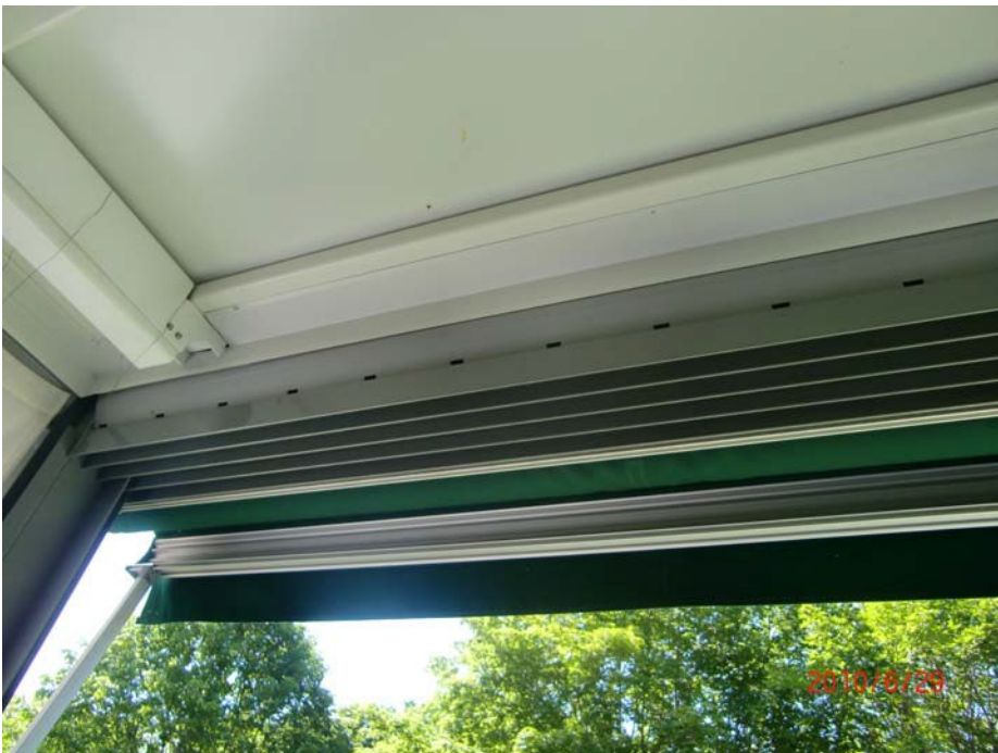
Picture 6. The sound insulation shows certain weaknesses at the point of contact with balconies above. See more in section 5 (Bellman)
