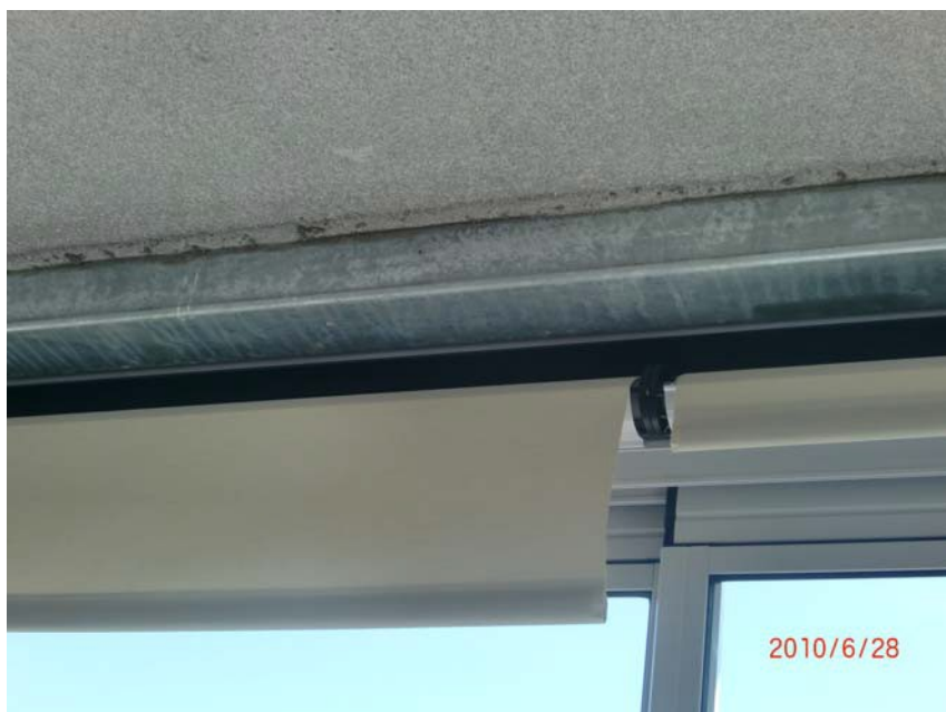
Picture 4. The sound insulation is weak at the point of contact with balconies above. See more in section 5 (Gaffeln)
